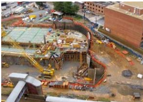
Photo from Montgomery County Construction of the Paul S. Sarbanes Silver Spring Transit Center is on schedule for an October 2011 opening. Upon completion, it will be one of the busiest transit centers in Maryland.
